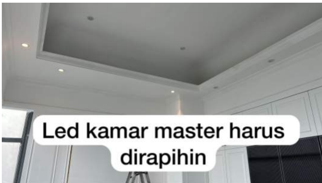
Gambar 4.2.6 lampu led kamar master Sumber : foto pribadi
