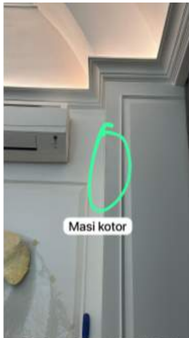
Gambar 4.2.8 wall panel defect Sumber : foto pribadi
