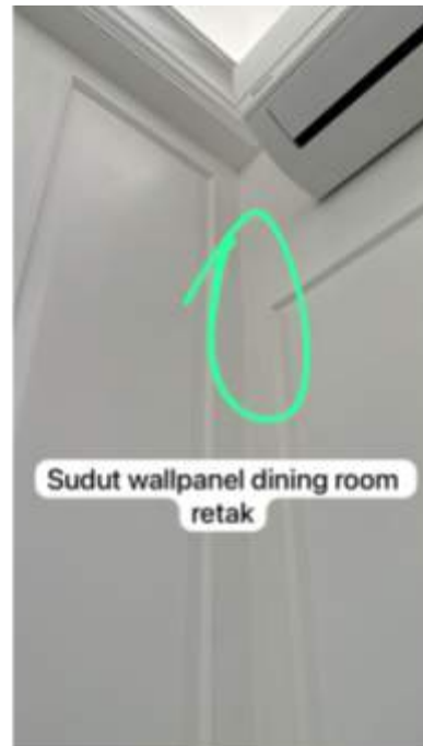
Gambar 4.2.9 wall panel defect Sumber : foto panel
